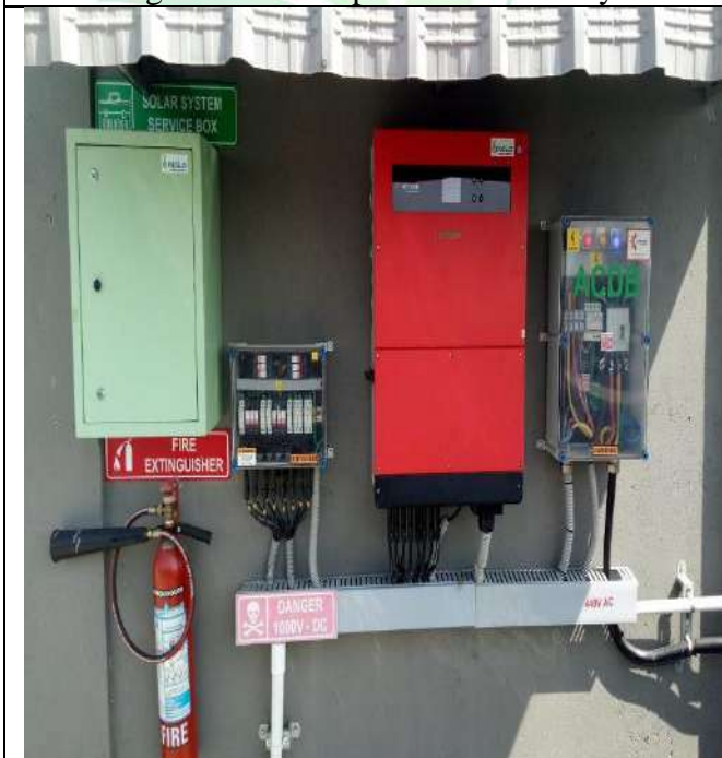
Figure 25: Solar system with Service box
