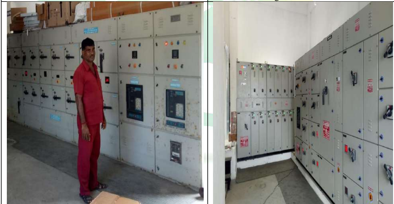
Figure 32: Power house Control Panels
