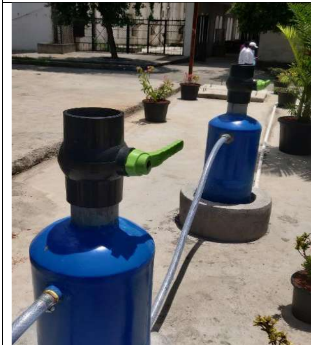
Figure 70: H 2 S Scrubber
