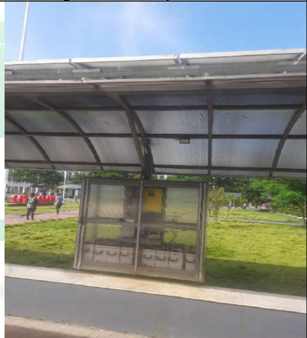
Figure 22: Solar Inverter with controller
