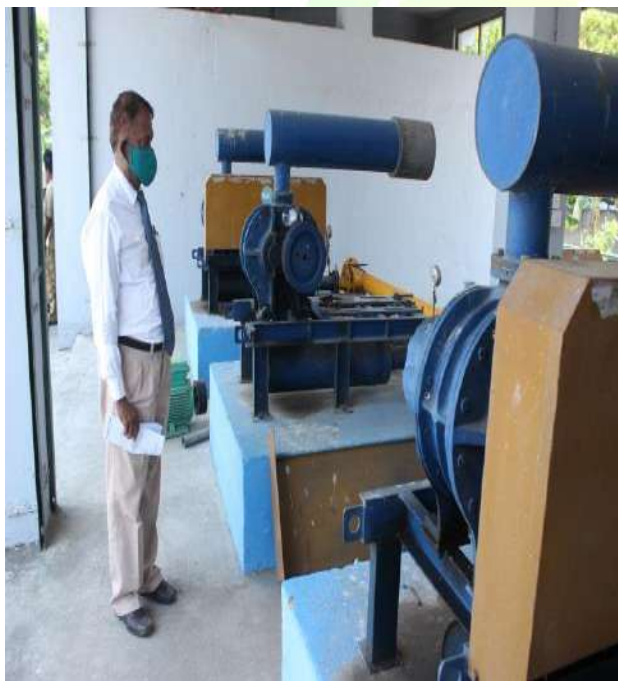
Figure 41 :Lead auditor inspecting the blowers
