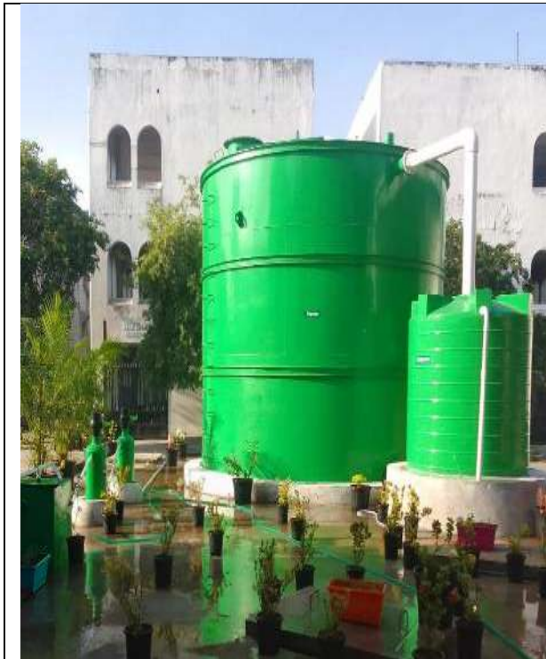
Figure 68: Biogas Digester and Slurry collection Tank
