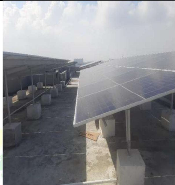
Figure 21: Rooftop Solar Panel
