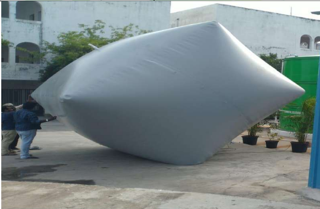
Figure 74: Biogas Storage Balloon
