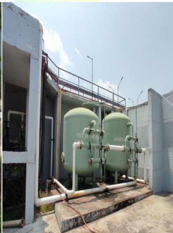
Figure 38: Water treatment unit
