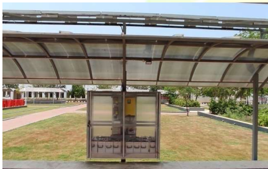
Figure 46: Solar panels with controller
