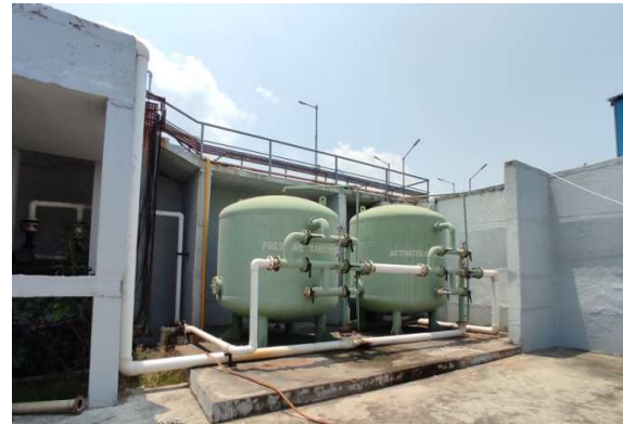
Figure 8: Water treatment unit
