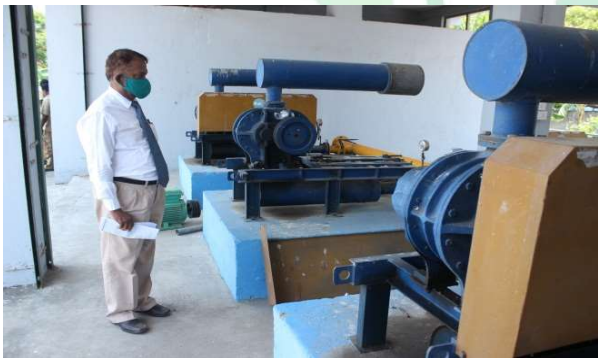
Figure 11: Lead auditor inspecting the blowers
