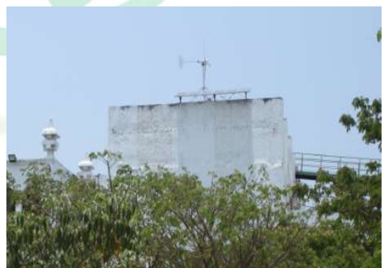
Figure 49: Solar-Wind Hybrid system
