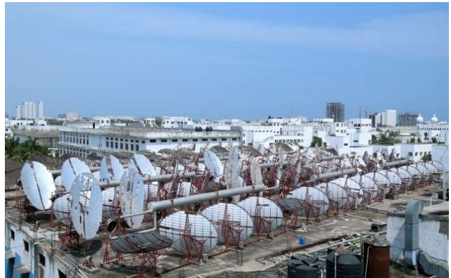
Figure 14: Solar cells on roof top
